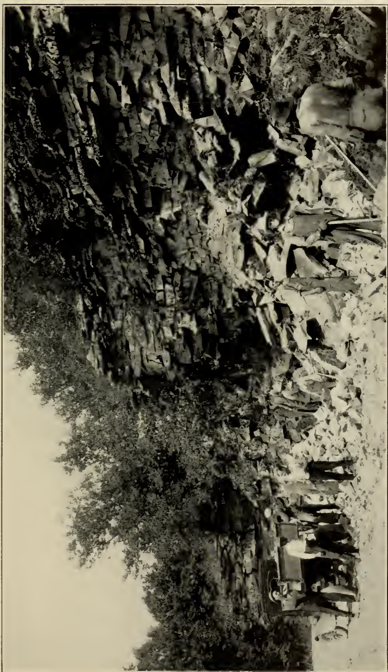
PLATE LIII.—Droop Sandstone of Manch Chunk Series on West side of Droop Mountain. Here it is fractured and broken, making suitable material for a road base for which it is being used. (Photo, by Paul H. Price).
